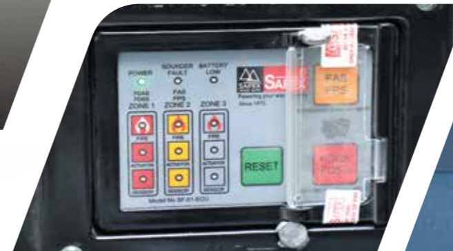
FAPS Control Panel
