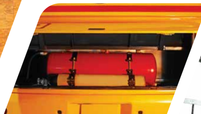
Water Tank And Nitrogen Tank
