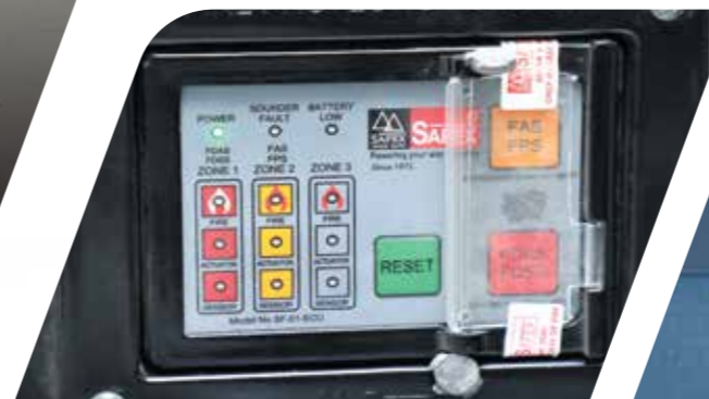
FAPS Control Panel
